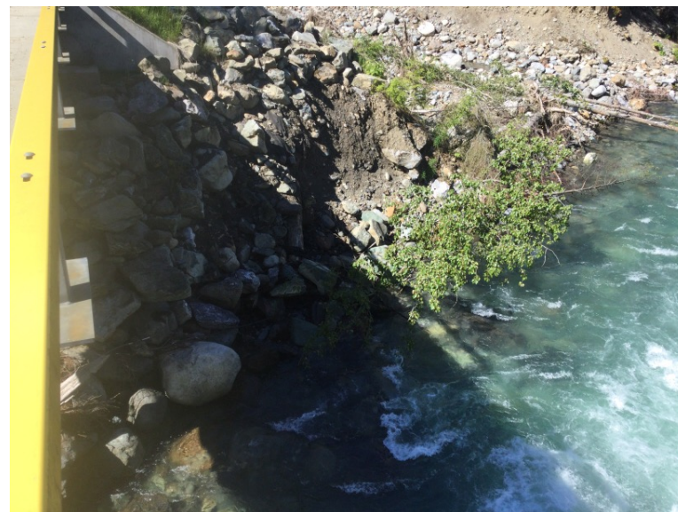
Downstream left bank riprap erosion
