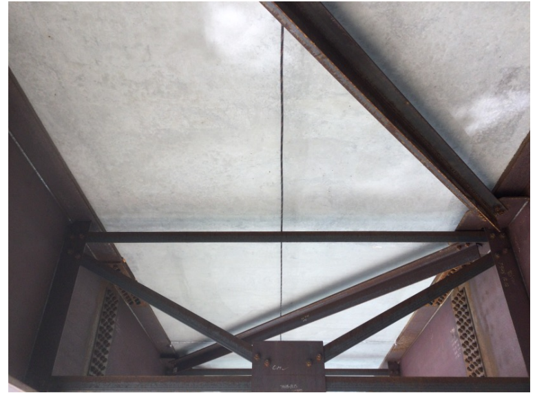
Cable access under deck
