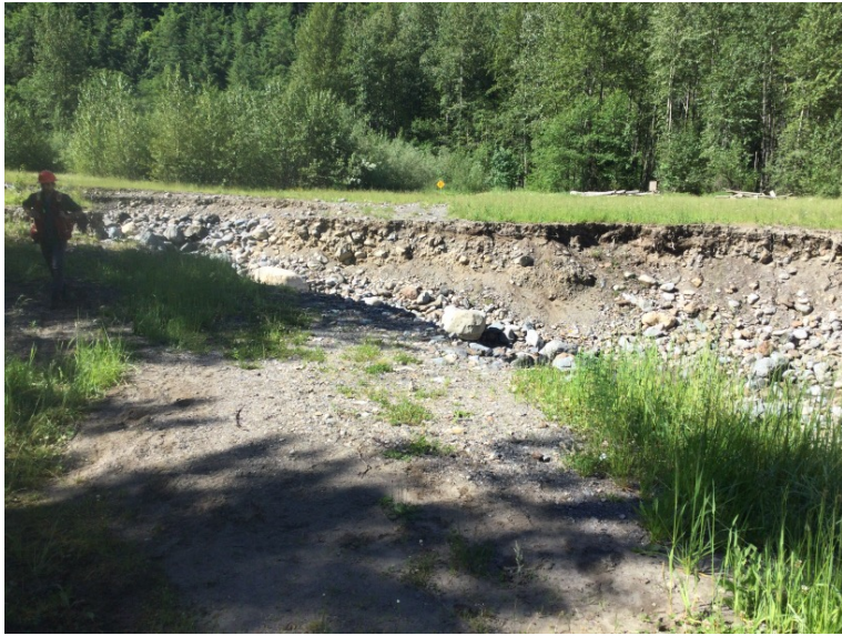
Looking at left bank approach subgrade erosion
