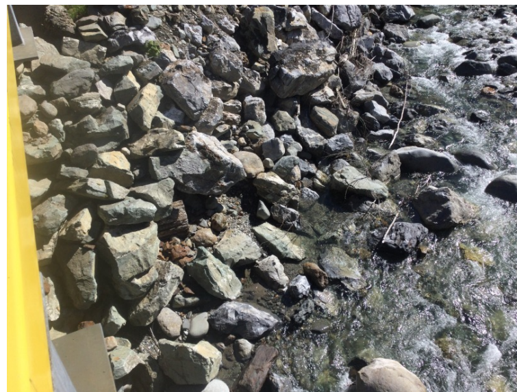
Upstream right bank riprap erosion
