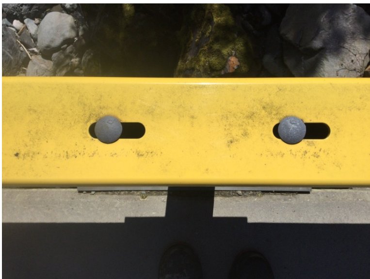
Plate washers not installed on rail
