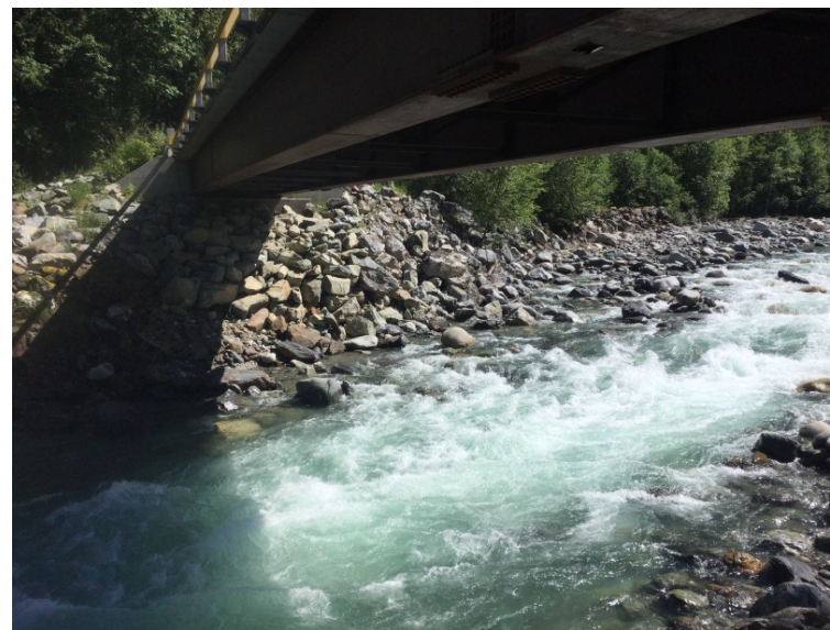
Upstream right bank riprap erosion
