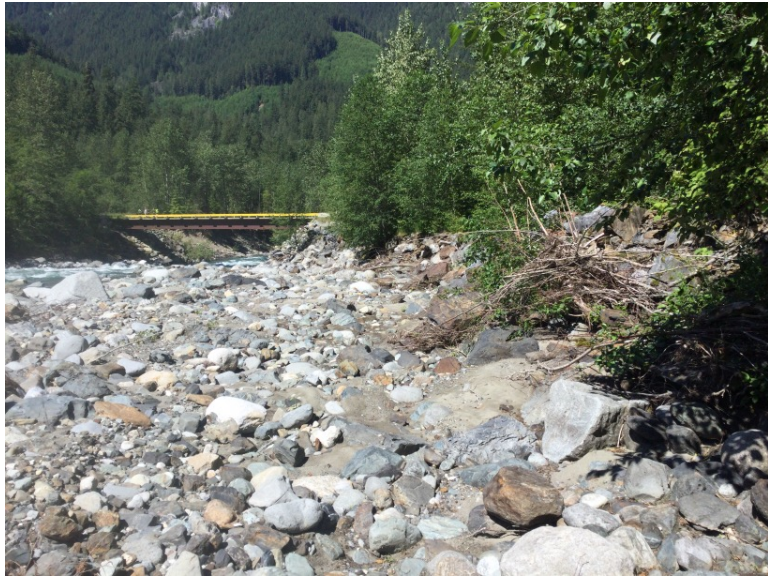
Upstream right bank Riprap erosion extent -100m extent
