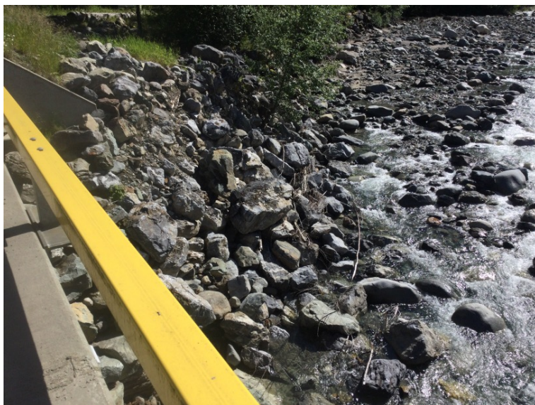
Upstream right bank riprap erosion
